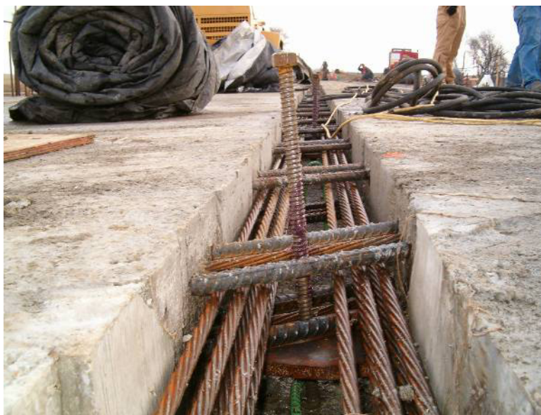
Figure 34. Longitudinal joint congestion on Boone County Bridge
